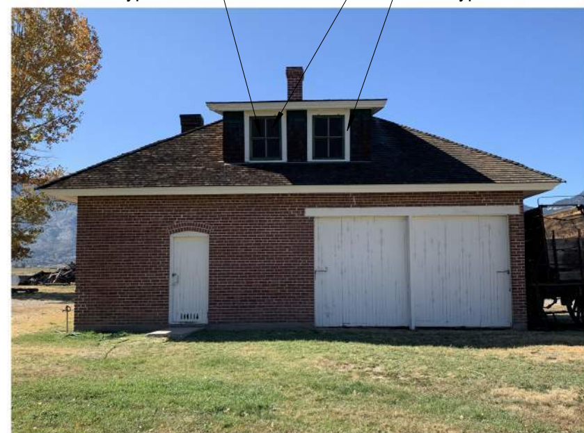
D5 Photo of Existing Conditions Not to Scale
