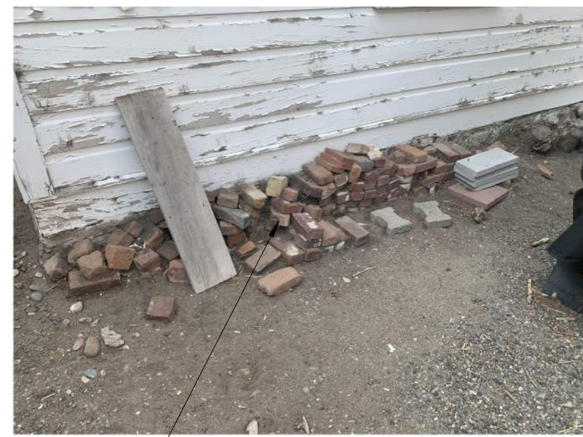
Portion of existing brick to utilize for rebuilding the Gateway Entry coordinate with Dangberg Ranch Curator for quantity and location of existing brick
